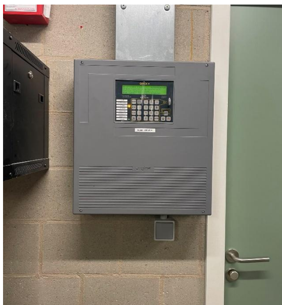
Brandcentrale in de kelder
