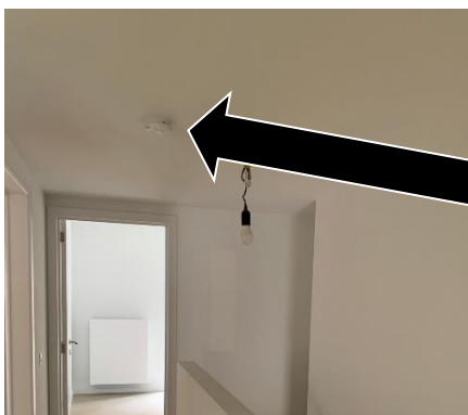
Rookmelder in appartement
