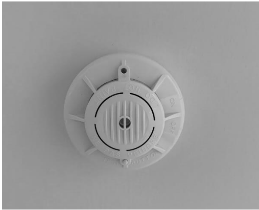
Rookmelder in appartement
