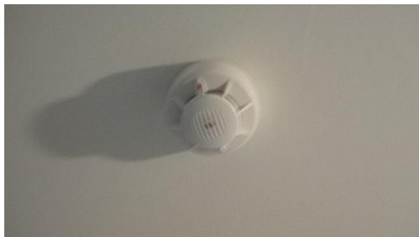
Rookmelder in appartement
