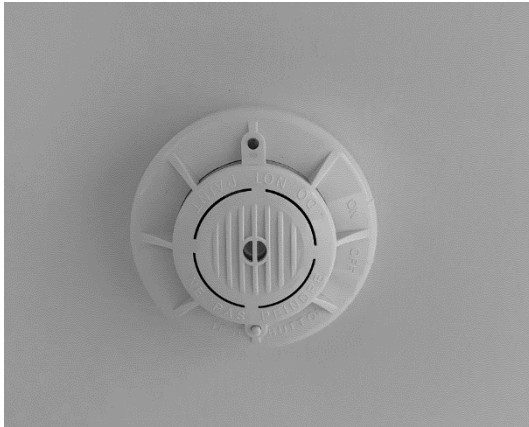
Rookmelder in appartement
